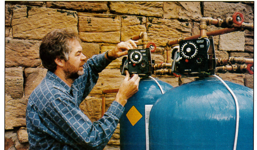
Eric Dalton puts the finishing touches to a new system installed on Lord Ingleby's Ripley Estate.
